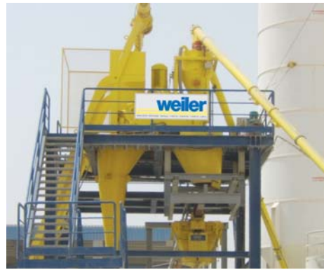
Batching plant with 2 discharge gates
